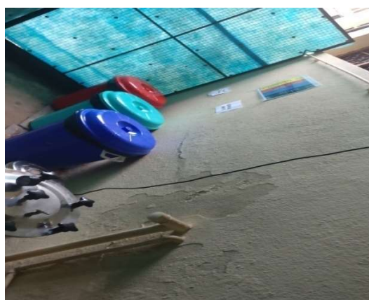
Image 23: Storage Room with no roof
