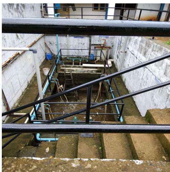
Image 11: Effluent Treatment Plant
